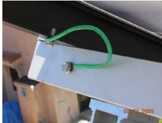
Connection of dissimilar (incompatible) materials
