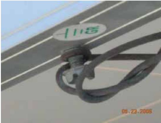
Poor installation connection
