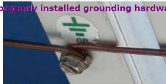
Dry-location lug rusting outdoors
